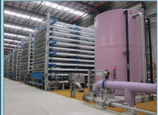
RO Facility, Perth Source: CH2M
