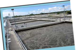
Aeration Basin Bacteria eat the dissolved solids and denitrify ammonia into nitrogen gas.
