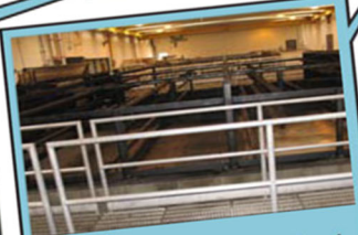
Thickening Sludge is thickened and de-watered before it goes to the digester.
