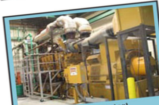
CoGen Facility (Generator) Methane gas is burned to create electricity that runs our plant.
