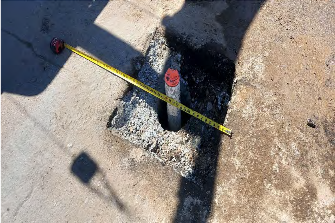
No. 24 – Monitoring well condition at time of City of Albuquerque inspection prior to concrete placement.
