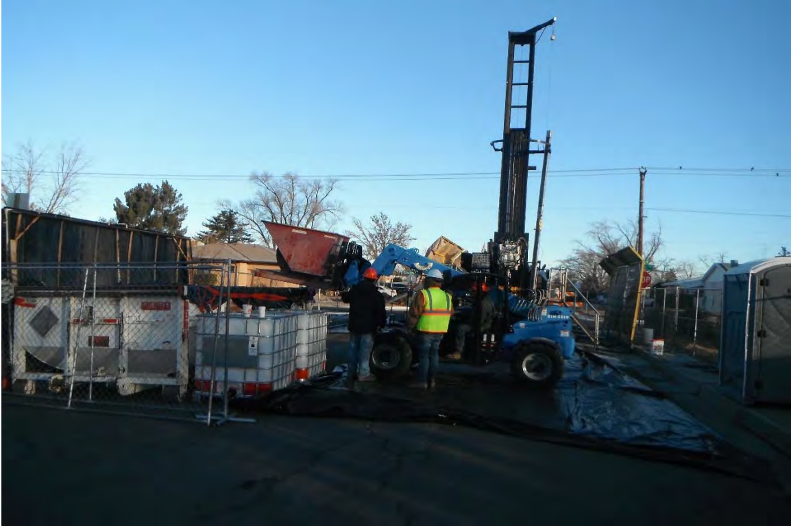
No. 7 – Photograph of dumping hopper (cuttings from rig to roll-off).
