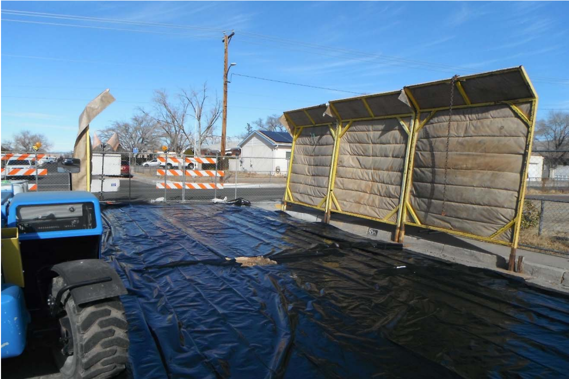
No. 4 – Daylighted boring/plastic placement, and sound panels prior to parking drill rig.
