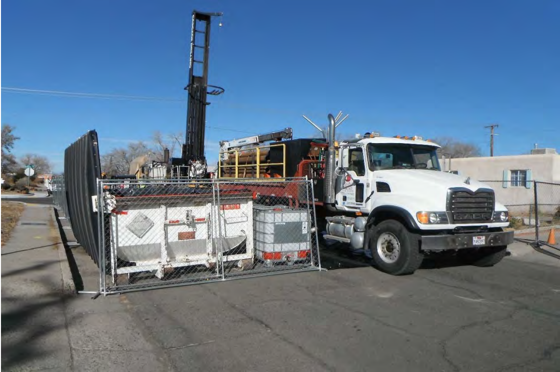
No. 5 – Layout of drill site with roll-off, totes, and support truck with drill casing.
